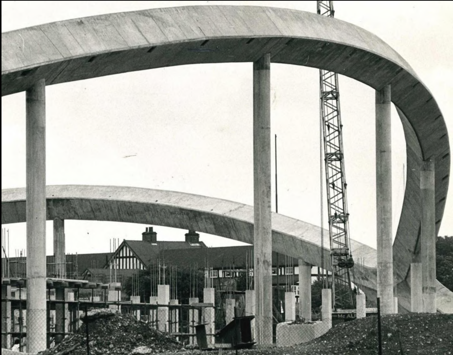
The elliptical concrete arches of the pioneering roof at the Richard Dunn Sports Centre, under construction in 1975.
